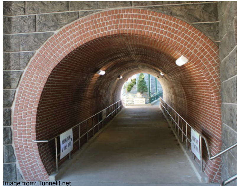
Image from: Tunnelit.net Potential Solution
